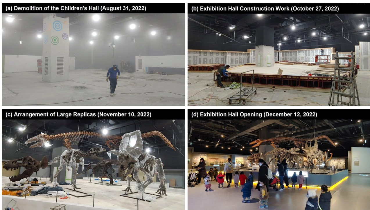
Fig. 2. Construction process of the ‘Evolution of Life’ Hall at the Daegu National Science Museum.
