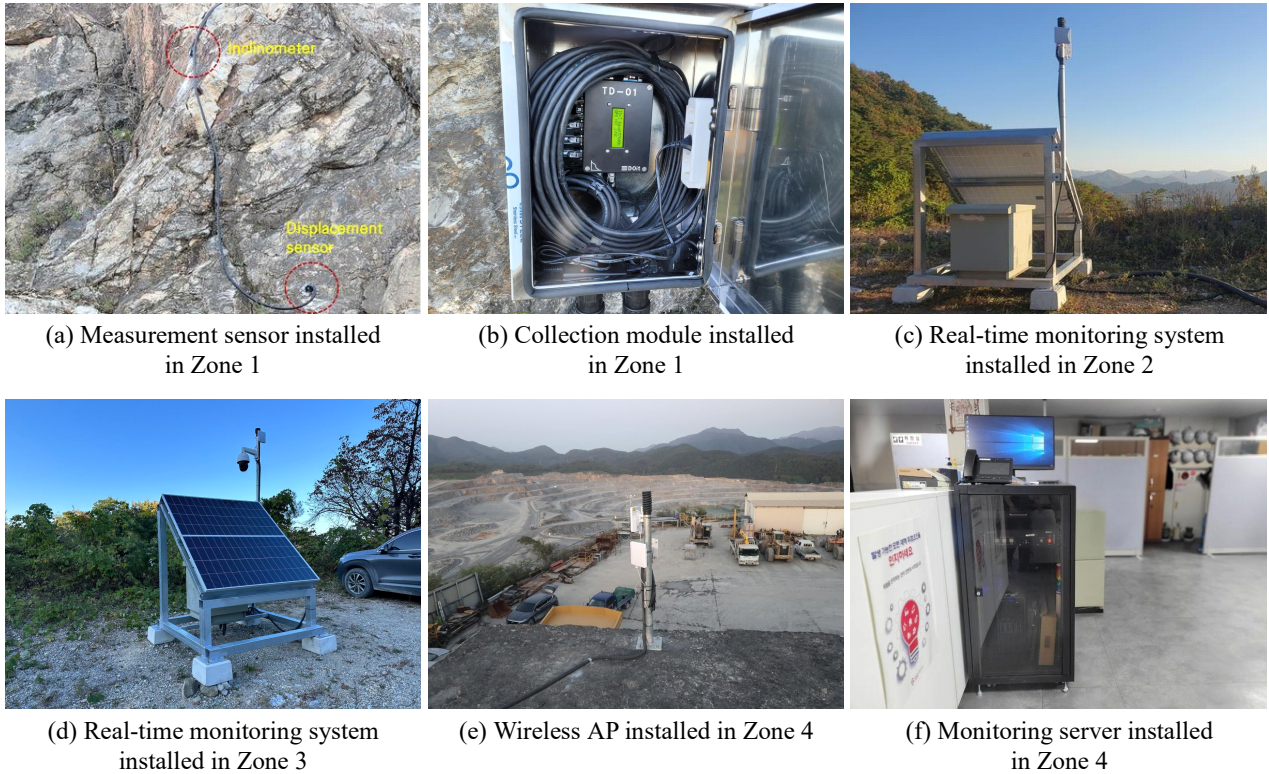
Fig. 9. Real-time monitoring system built for field performance evaluation.
