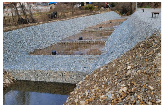
Fig. 2. A view of pretreatment system.
