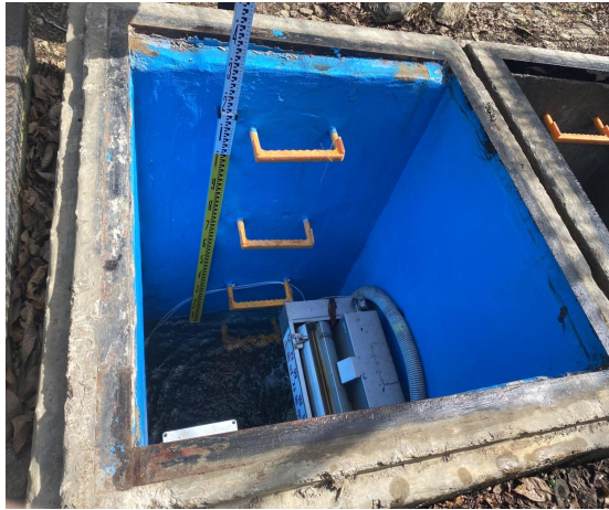
(a) Water tank level measurement using staff
